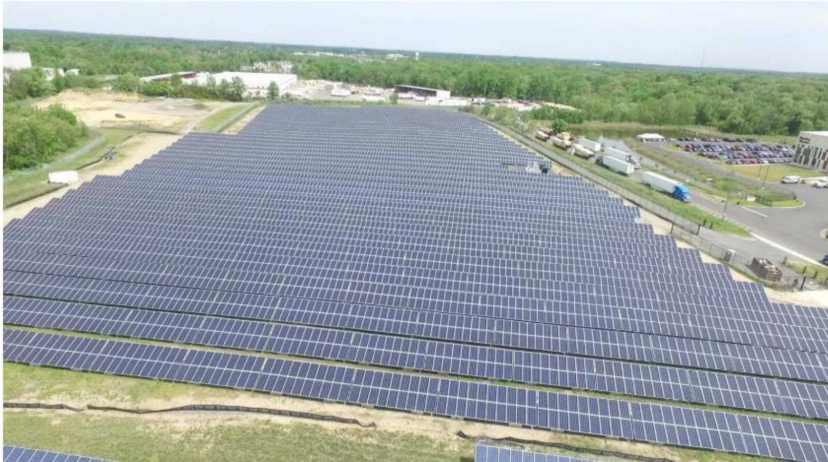
Tri-County Landfill Solar Farm, Delanco – Soltage/AC Power
